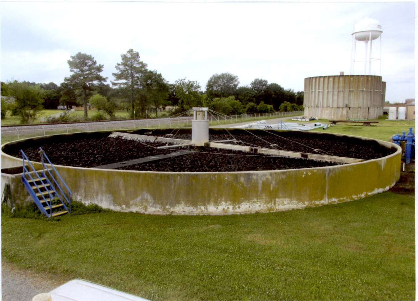
5. OPERATING TRICKLING FILTER
