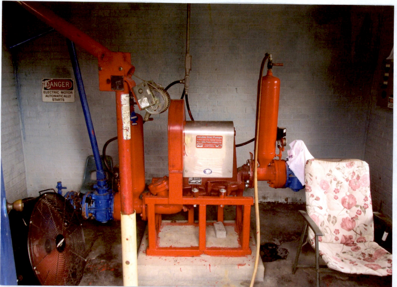
4. PENN VALLEY PRIMARY SLUDGE PUMP
