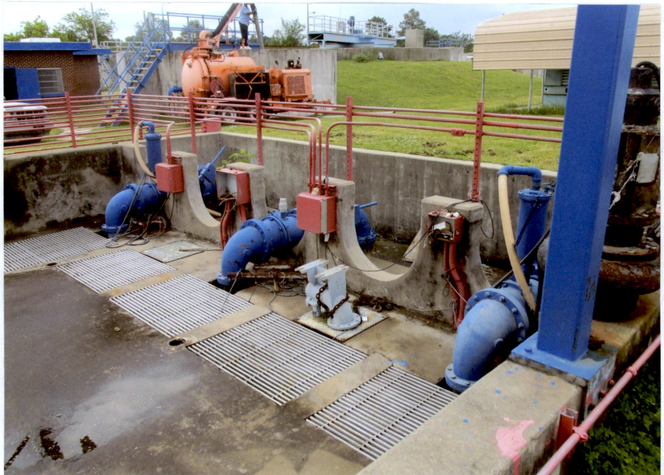
2. PRIMARY PUMPING STATION - A PUMPS TO TREATMENT
