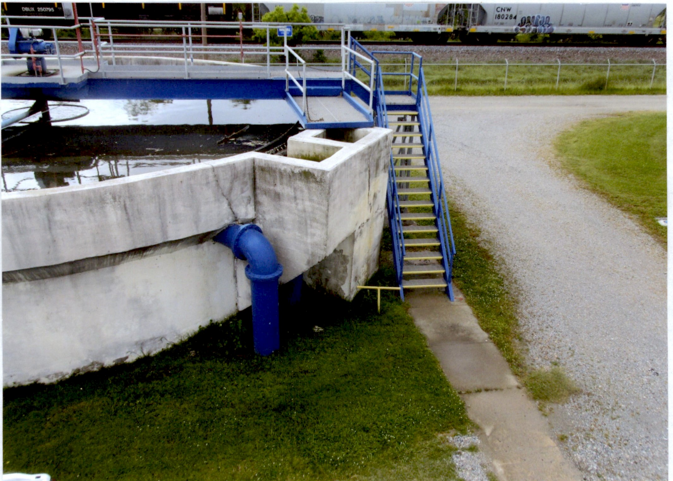
4. MID SIZE PRIMARY CLARIFIER
