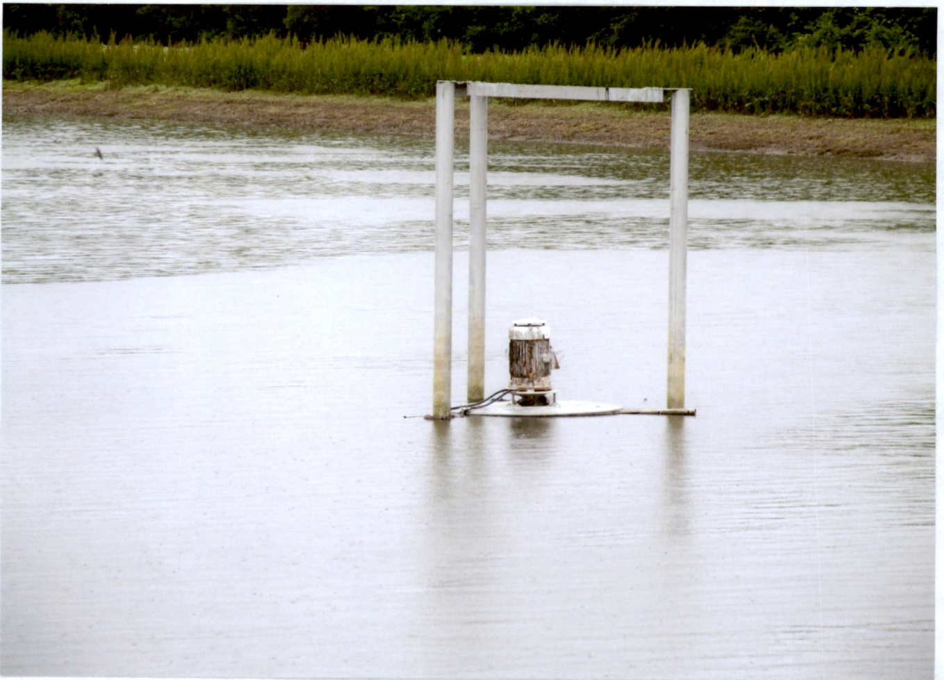
14. SOUTH AERATOR IN FLOW REGULATION POND TO BE REPAIRED
