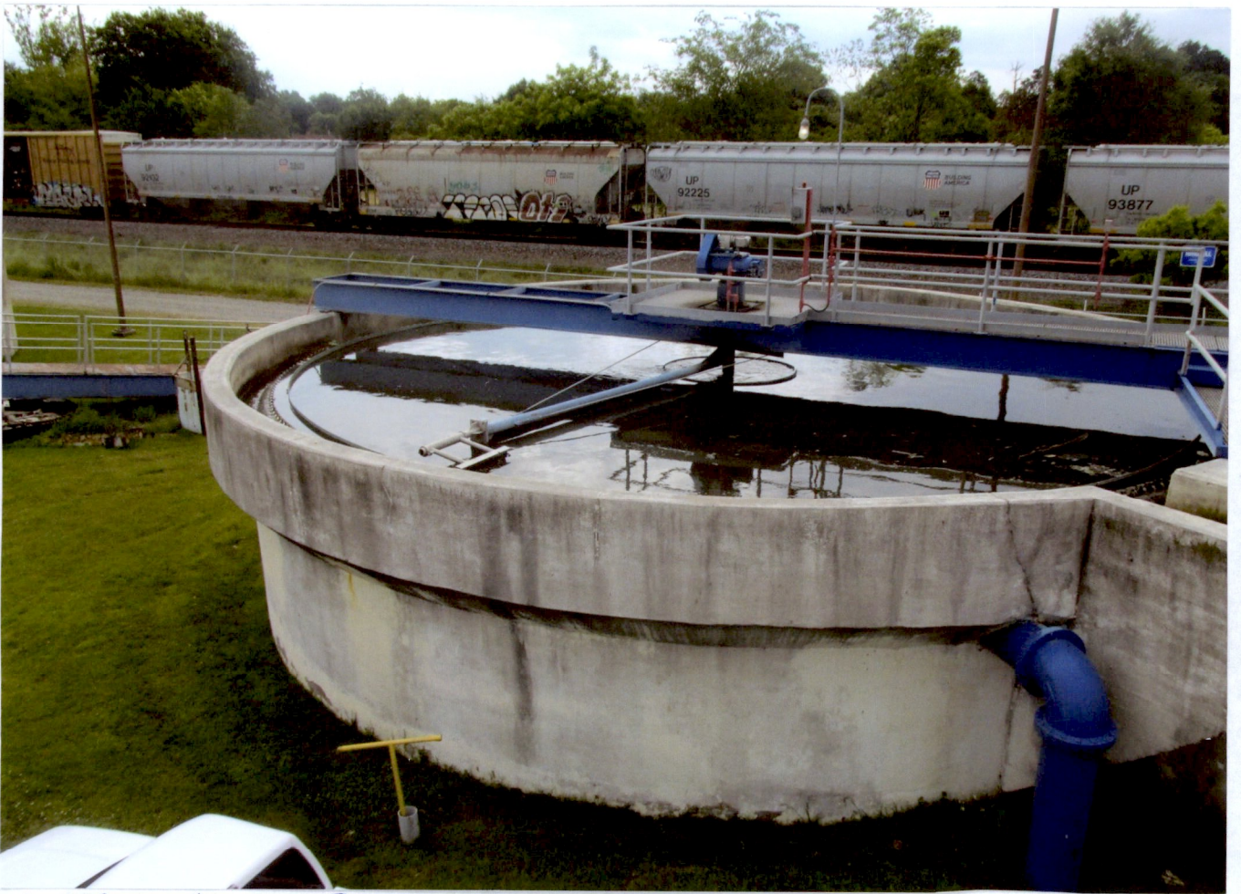
4. MID SIZE PRIMARY CLARIFIER
