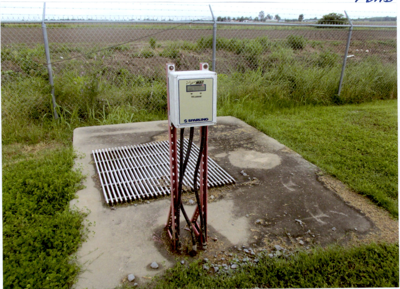
2. PRIMARY PUMPING STATION- FLOW RECORDER
