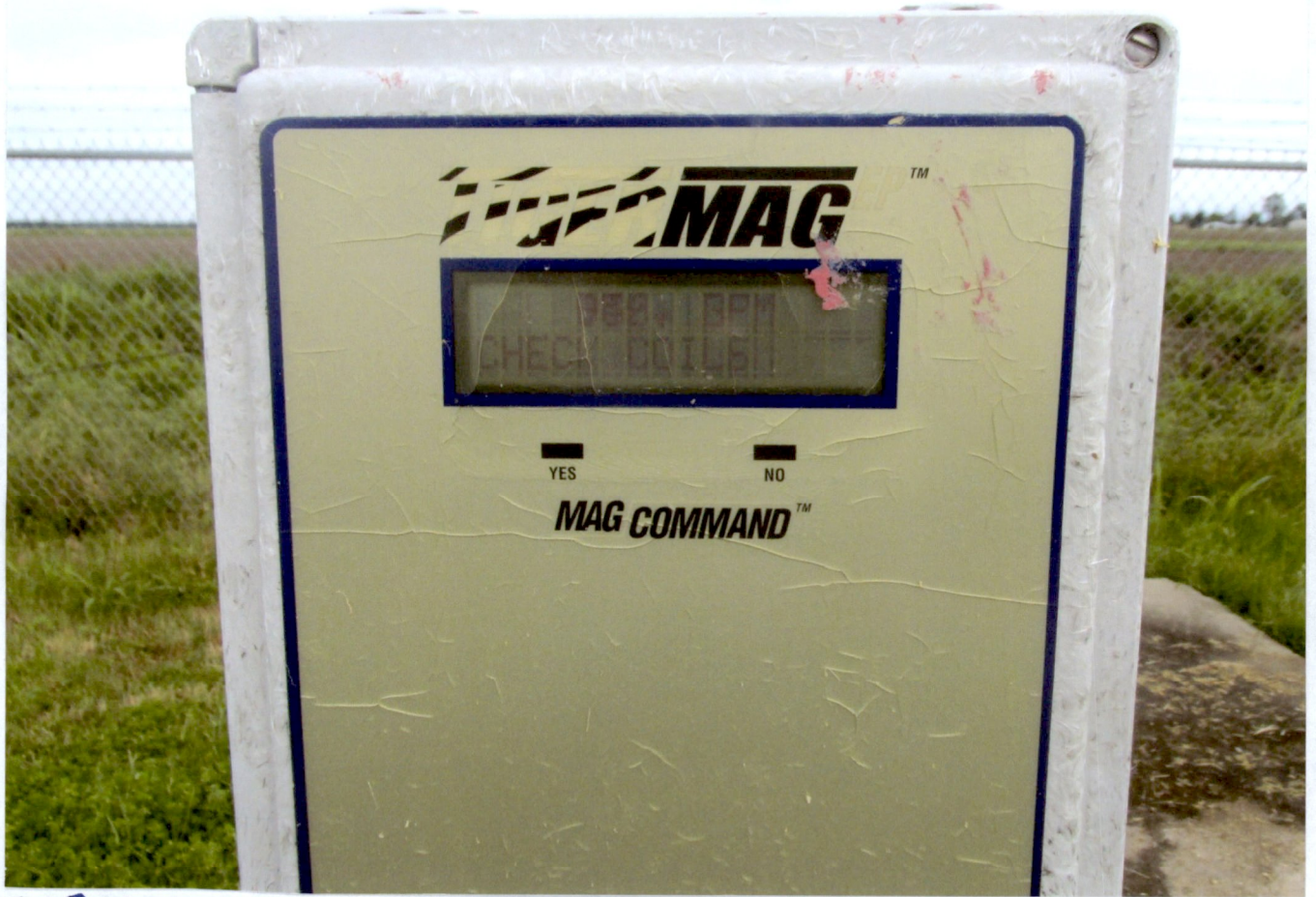
2. PRIMARY PUMPING STATION - FLOW RECORDER
