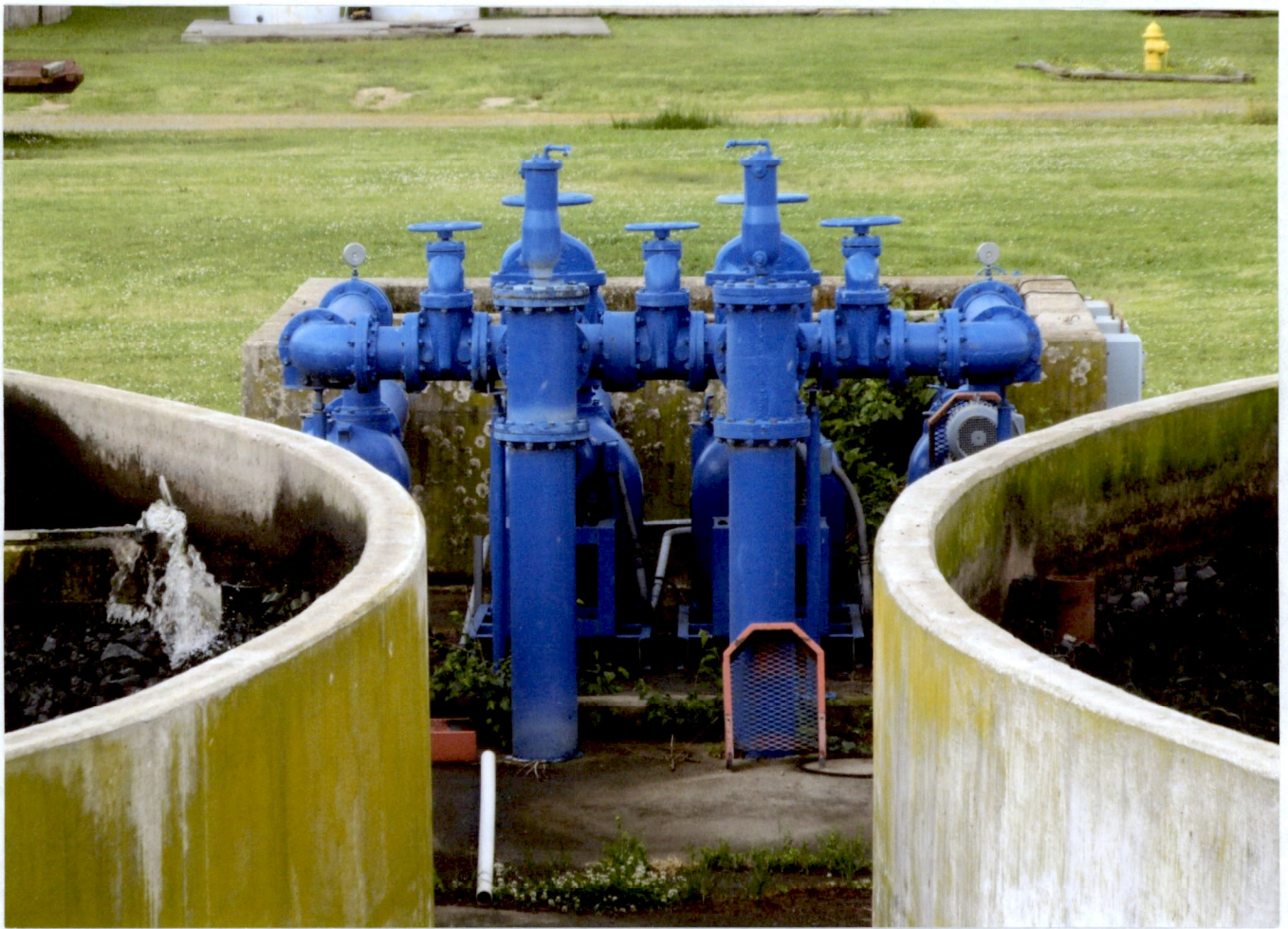
5. TRICKLING FILTERS RECIRCULATION PUMP STATION 4TH PUMP REPAIRED AND BACK IN SERVICE
