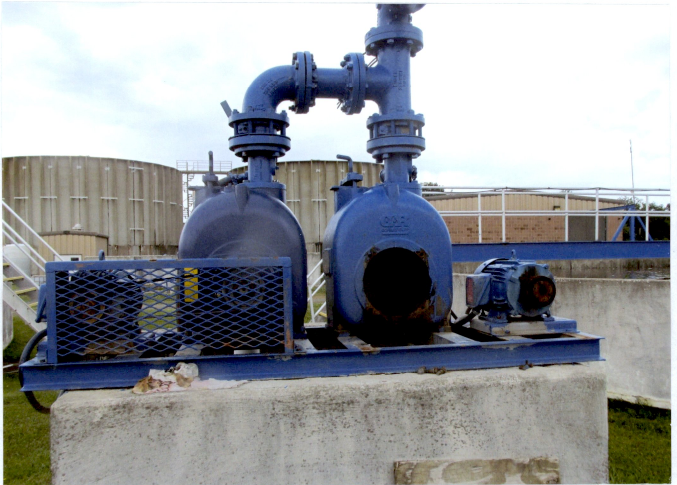
9. NORTH CLARIFIER PUMP STATION- DOWN FOR REPAIR
