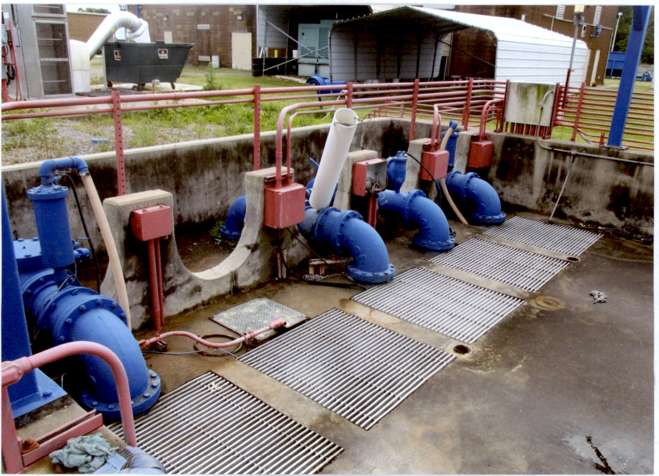
2. PRIMARY PUMPING STATION- 8 PUMPS TO FLOW REGULATION POND
