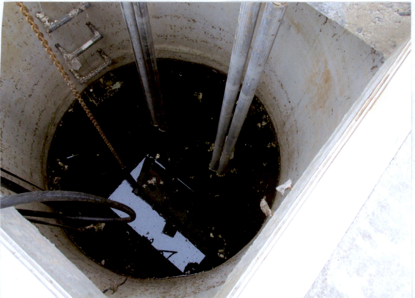
14. PUMP BACK PUMP STATION-LOOKING DOWN THRU MANWAY
